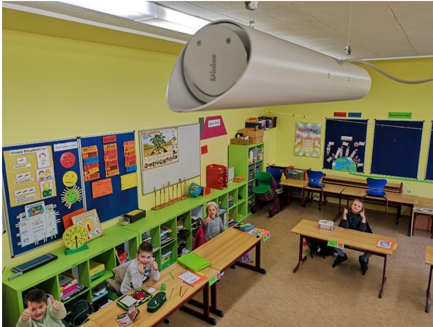
Image 1 Dinies UVG80 Air Disinfection in a classroom
